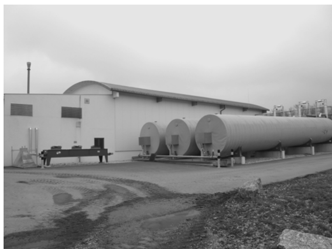
Photo 2. A view of steel tube fermenters 8 (right part of photo) – BGS Amstetten (Austria) – photo by authors
