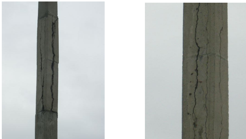
Figure 2. Cracks at some of the bridge concrete hangers
