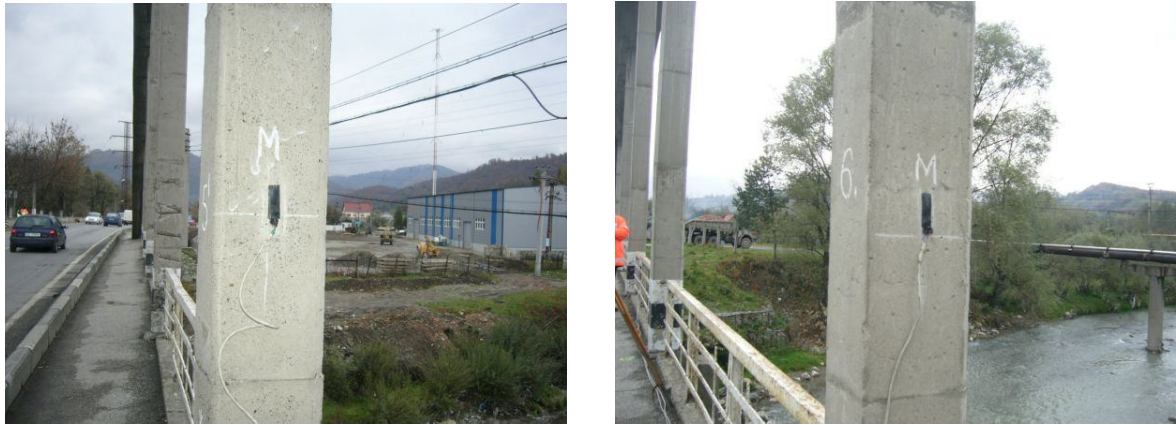
Figure 4. Electro-resistive transducers placed on the concrete hangers
